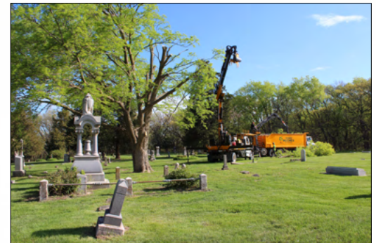
Paul Dietze, Certified NE Arborist, Jon Mason and Cody Lewis, Hughes Tree Service remove hazardous/defected tree located in the Elkhorn Cemetery founded around 1840. The cost of repairing the tomb stones caused by the tree failure would have greatly exceeded the removal cost of the tree. (Jim Keepers photo)
